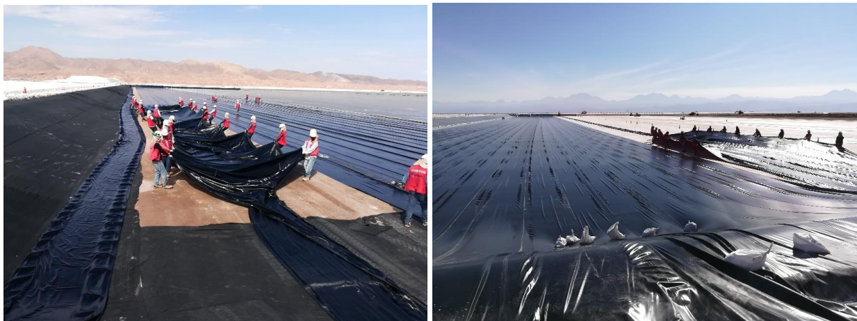
Figure 7. Photographs of unfolding geomembrane panel and allowing air under panel to pull it into proper location.
