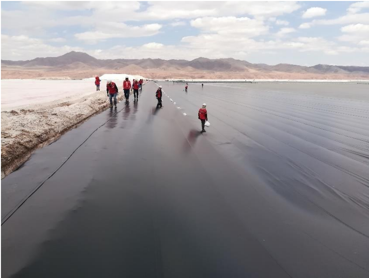
Figure 11. Completed liner system after deployment and field welding of geomembrane panels in desert environment.
